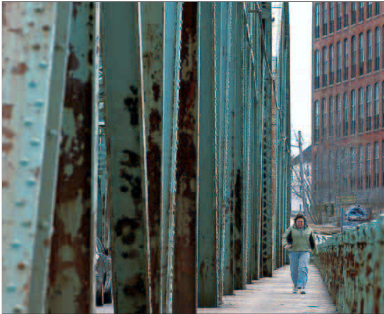
Colleen McKenna of Brunswick crosses the Frank J. Wood Bridge on Thursday in Brunswick. The state wants a path kept open on the bridge during repairs. The Androscoggin Swinging Bridge will close for repairs next week.
